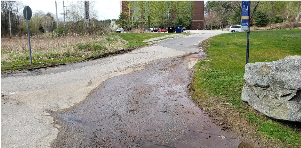
Photograph 8: Seepage observed on the Greggs Hall access road and Waterworks Road May 6, 2020
