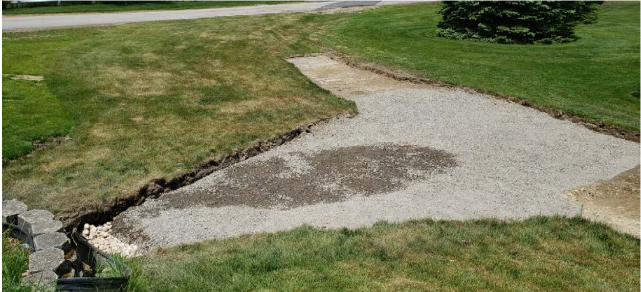
Photograph 7: View of Gundalow Landing seepage area following excavation and backfill with sand and gravel
